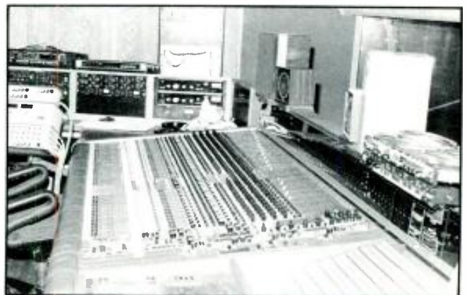
Accessory equipment lines racks to the left of the console.
